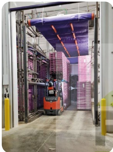
Above left: Forced air cooling tunnel observed during the California study tour.
