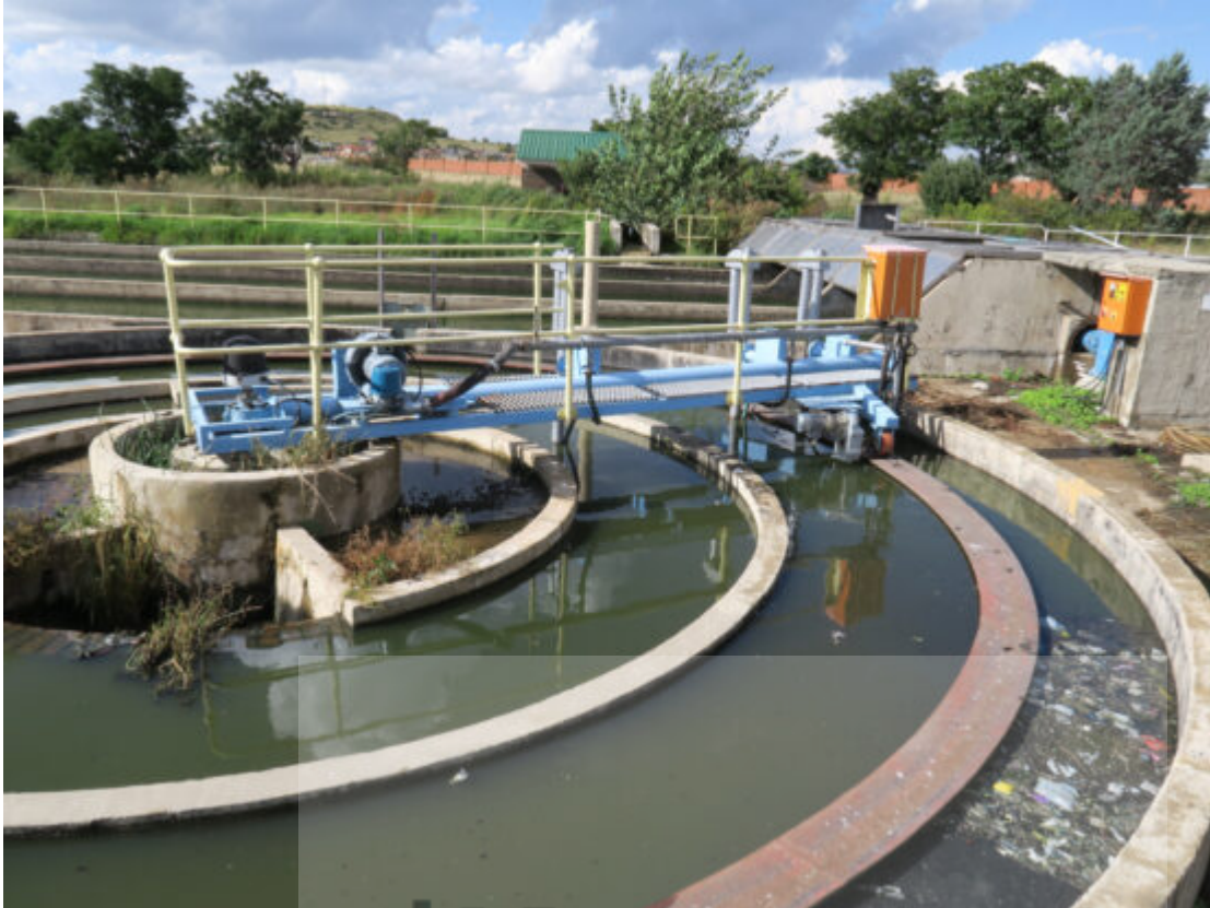
A dysfunctional sewage treatment works in Winburg, Free State, from which sewage flows untreated into the dam from which drinking water for the town is extracted. Image: Steve Kretzmann/GroundUp
