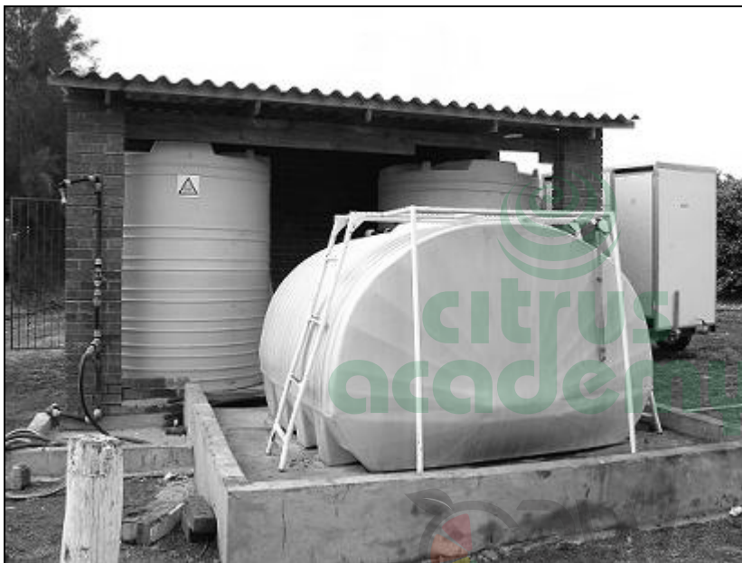
Figure 4.1: Fertigation Tanks at Crookes Brothers (Nkwalini)
